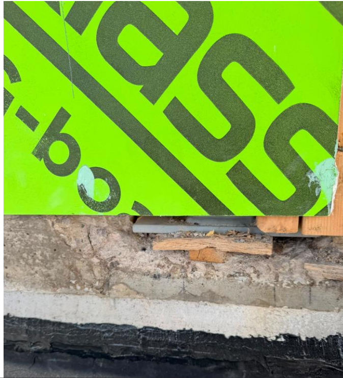
Timber packers to be removed and replaced with steel shims
