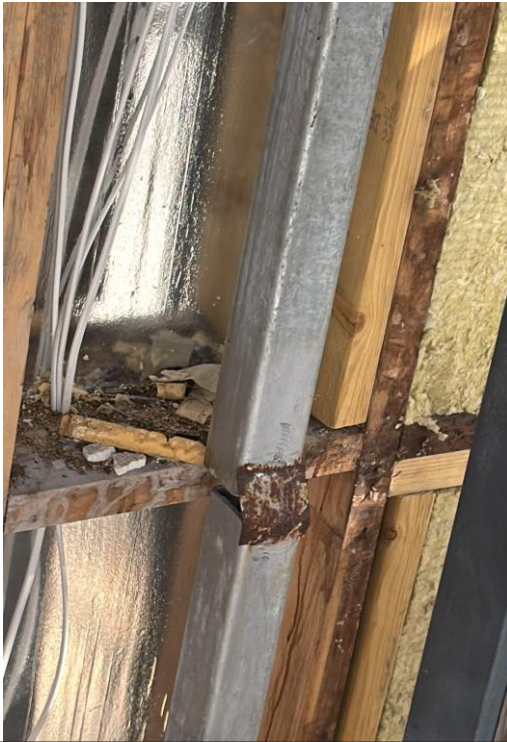
Re welding required to box section steels
